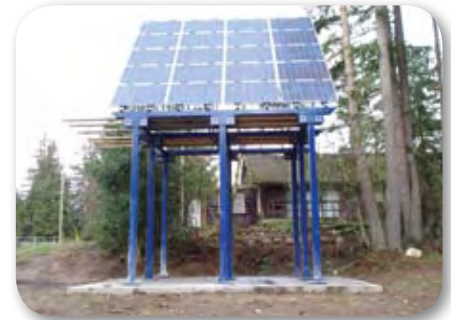
Net metering photovoltaic solar array in Anmore
