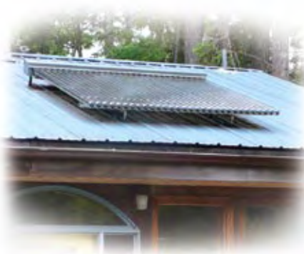
Solar Roof, Stone Glen Farm, Salt Spring Island
