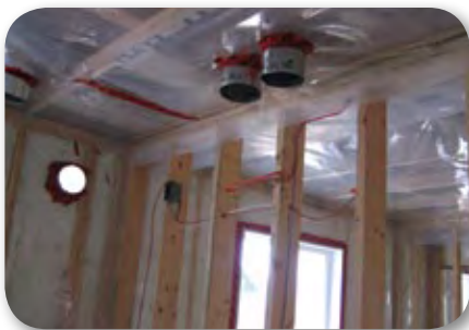
Insulation and Heat Recovery Vents in Kitamaat Village
